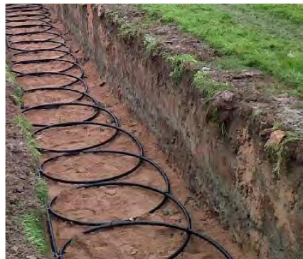
Ground Source Heat Pump
